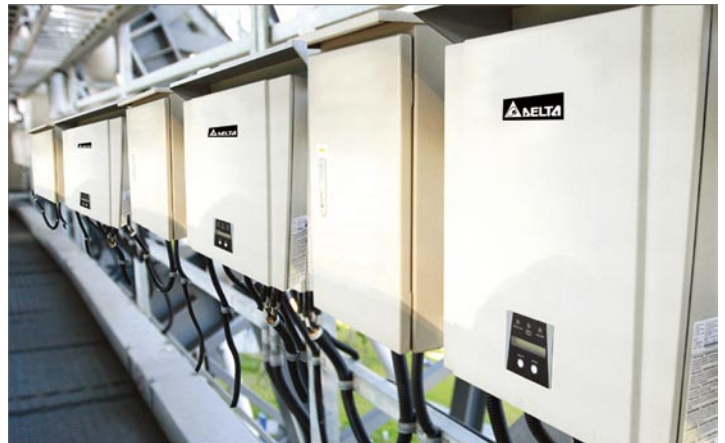
Photovoltaic Inverters Installed under Solar Panels
