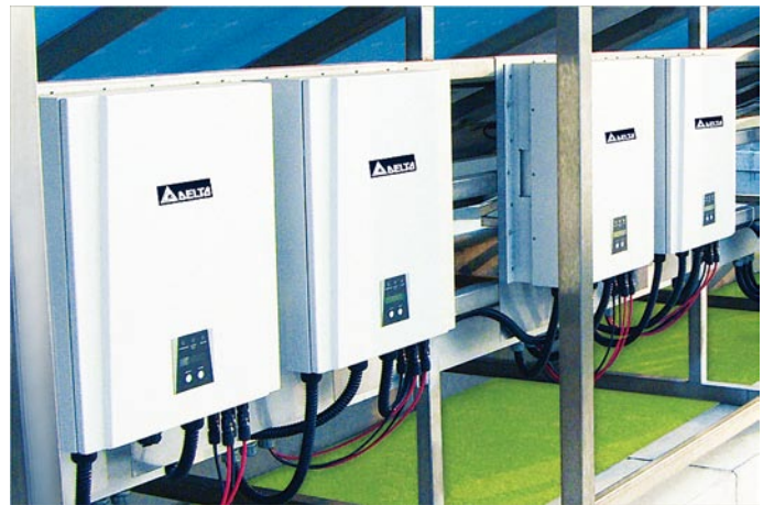
Photovoltaic Inverters Installed under Solar Panels
